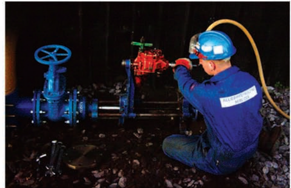
After pressure testing, the drilling machine is attached to the valve and the pipe drilled
