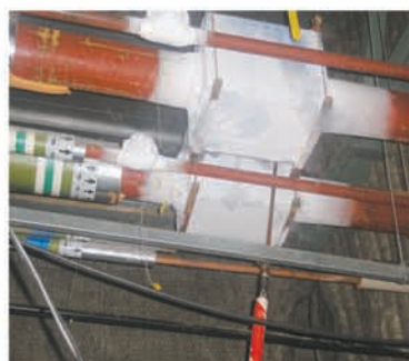
Once the jackets are sealed around the pipe, liquid nitrogen is pumped in to the jackets
